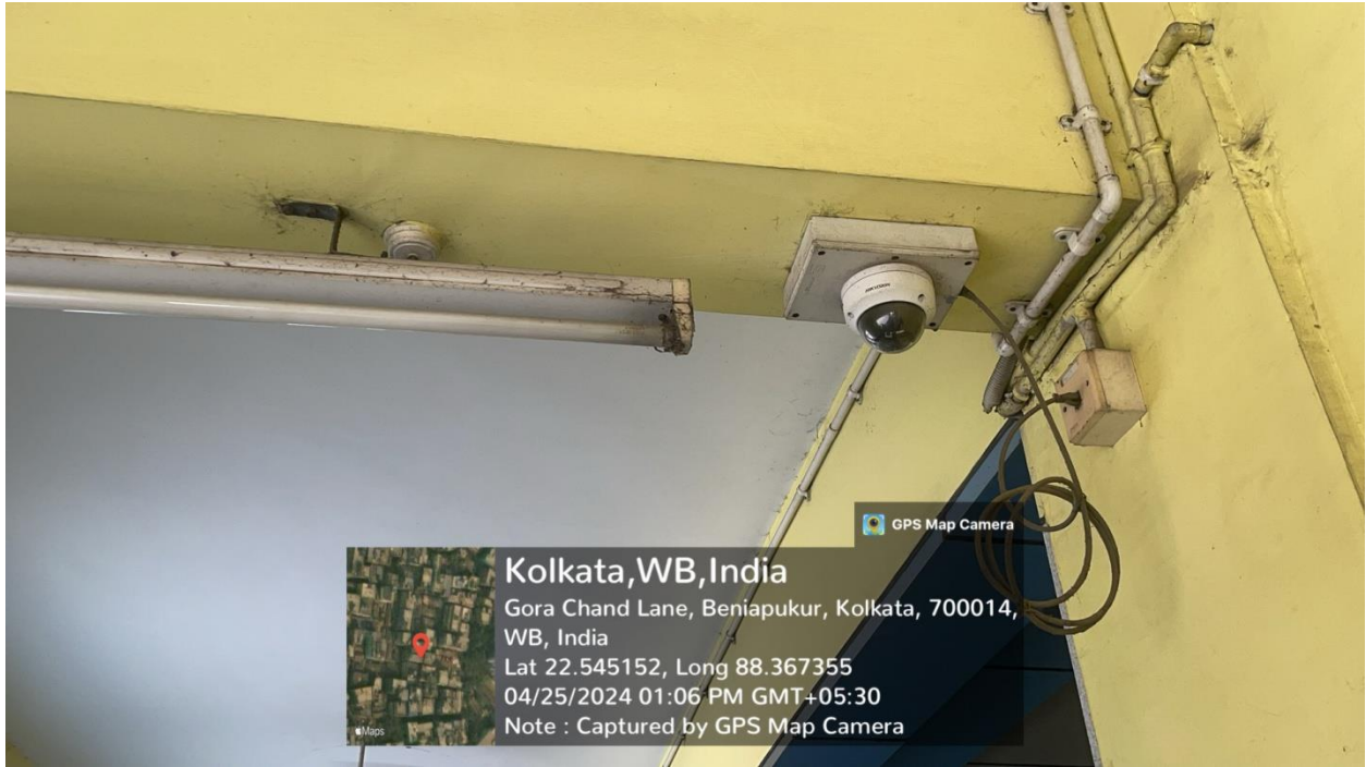
Figure 15: CC TV facilities
