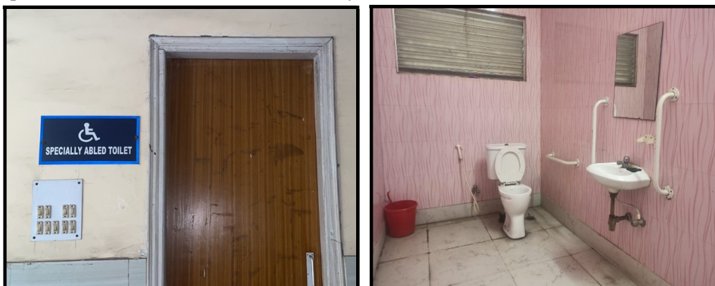
Fig. 7.1.7.2. Separate toilets for physically disabled candidates with special facilities
