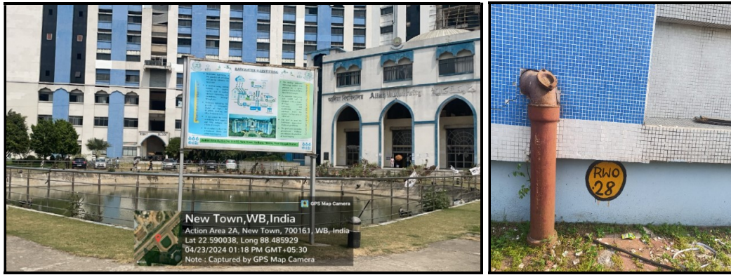
Fig.7.1.3.2: Rain water harvesting system at New Town Campus, Aliah University
