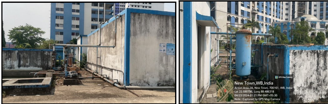
Fig.7.1.3.5: Waste water treatment and recycle plant at New Town Campus
