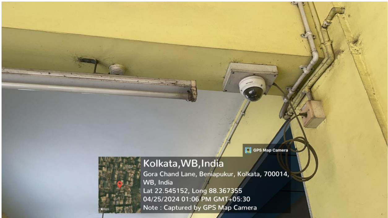
Figure 7: CC TV facilities
