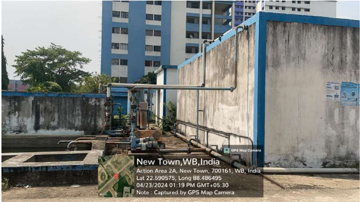
Figure 11: Water purification system
