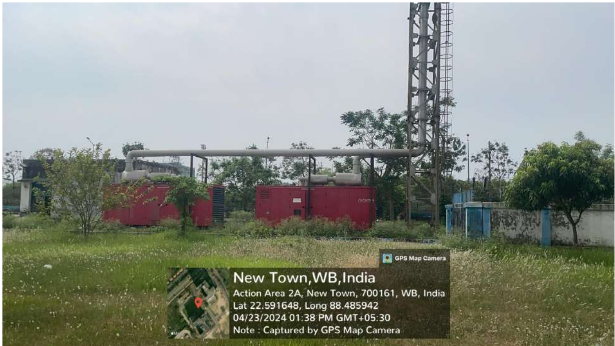
Figure 16: Generator facilities for emergency
